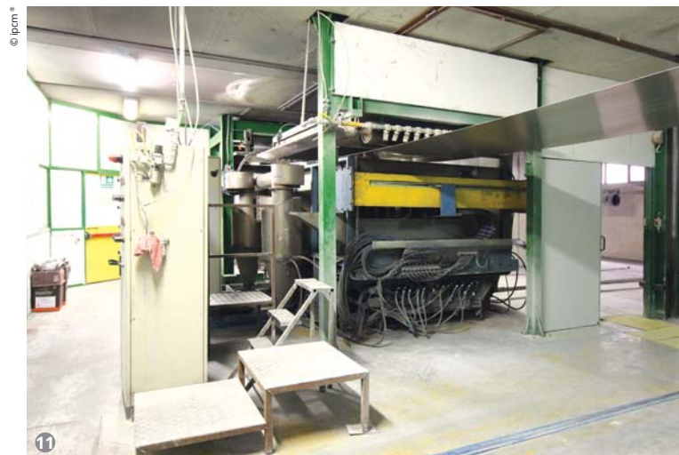
Figure 11: One of the two powder coating application booths.
