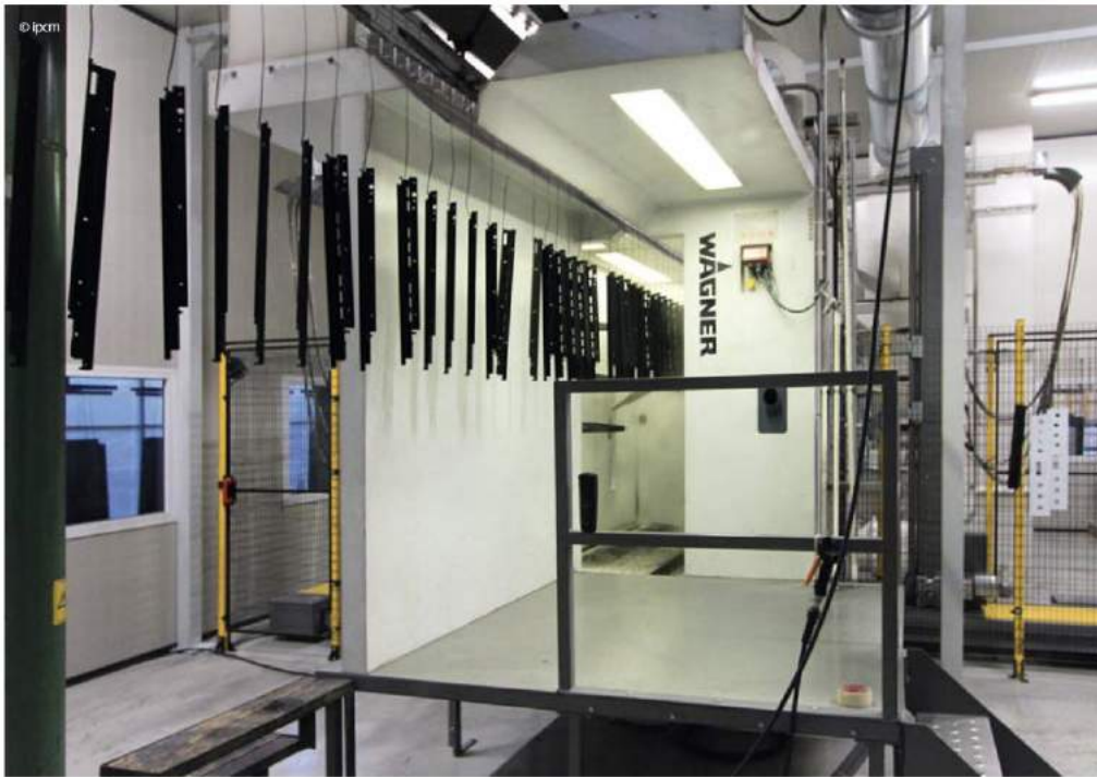
The new Wagner powder application booth.
