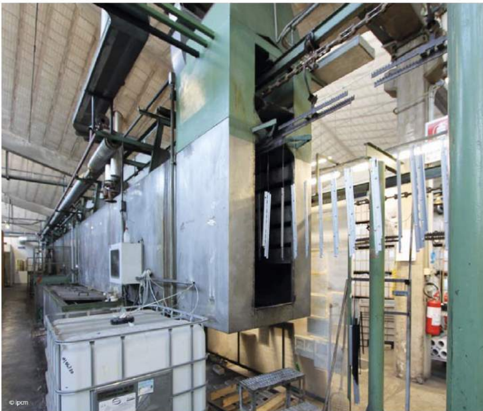
The pre-treatment tunnel.
