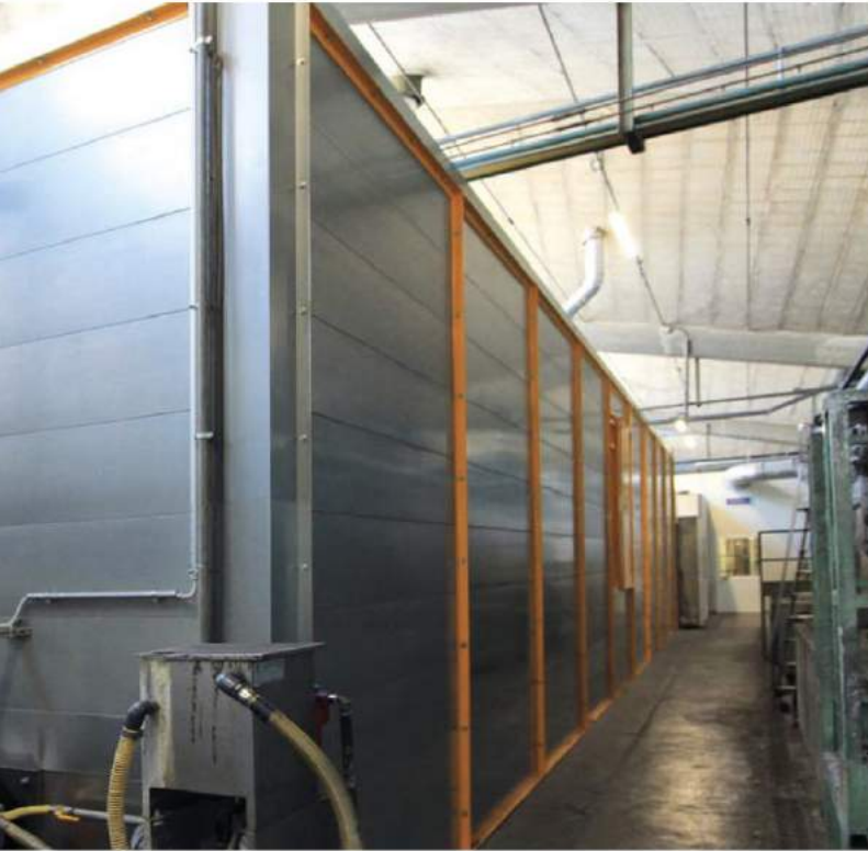
The new curing oven installed by Euroimpianti.
